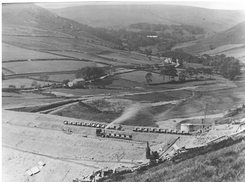
Figure 2: Fill placed on shoulder of the dam by side tipping from railway wagons
