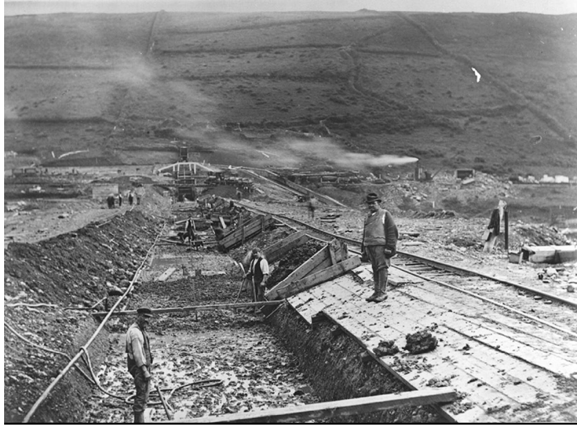
Figure 1: Puddled clay fill placed in cut-off trench up to level of dam foundation
